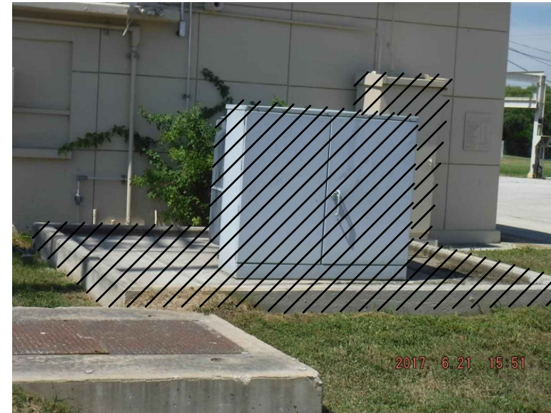
TRANSFORMER T-10 PHOTOGRAPH D 60DE01
