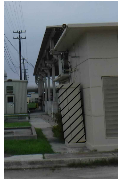
SWITCHBOARD SWB-6 PHOTOGRAPH C 60DE01
